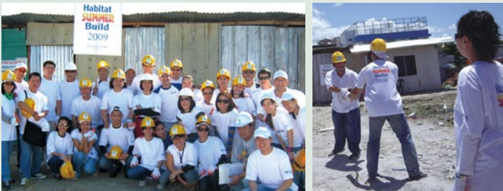
88 volunteers from The Peninsula Manila worked for 2 consecutive Saturdays to lay the foundation for one of the first houses to be built at a new Habitat for Humanity site in Nagpayong, Pasig City.
